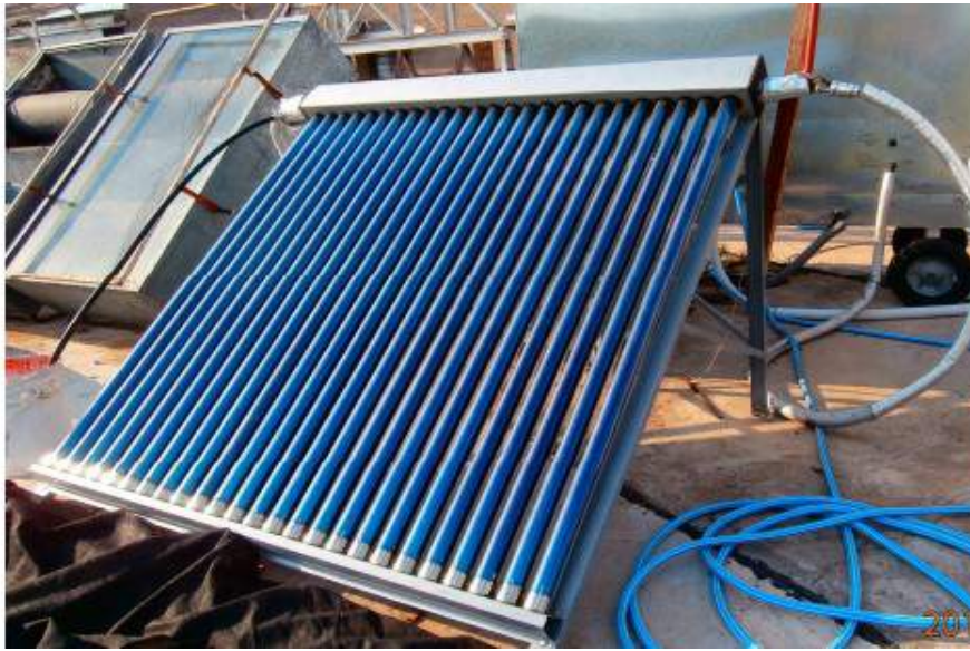
Figura 1. Colector de tubos evacuados “water in glass”
